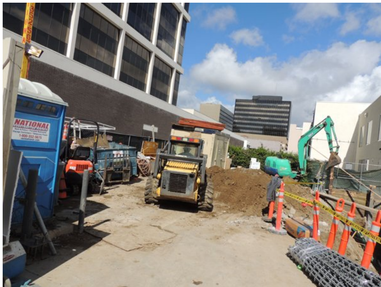
BEFORE THE GLITTER: Construction crews work on the space of what will become the Burberry building on the corner of Rodeo Drive and Dayton Way.
